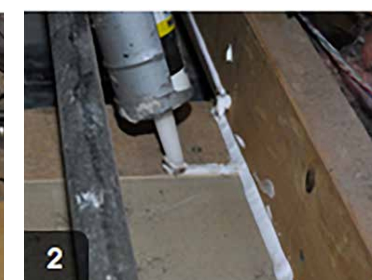
2 Sealant should extend along surround joist and into seams at top plates
